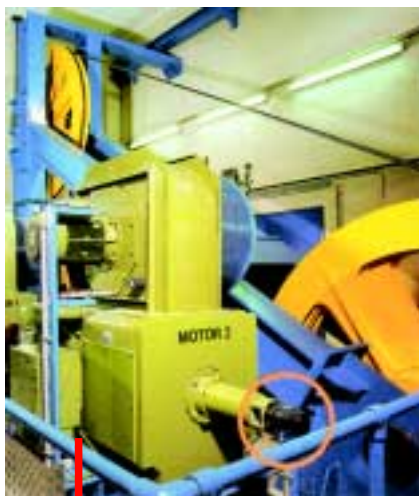
Figure 14: Tachogenerators with own bearings form a rugged unit with the driving machine (here a TDP 0,2 on one of the 500 kW drives of the Zugspitz cable-car).
